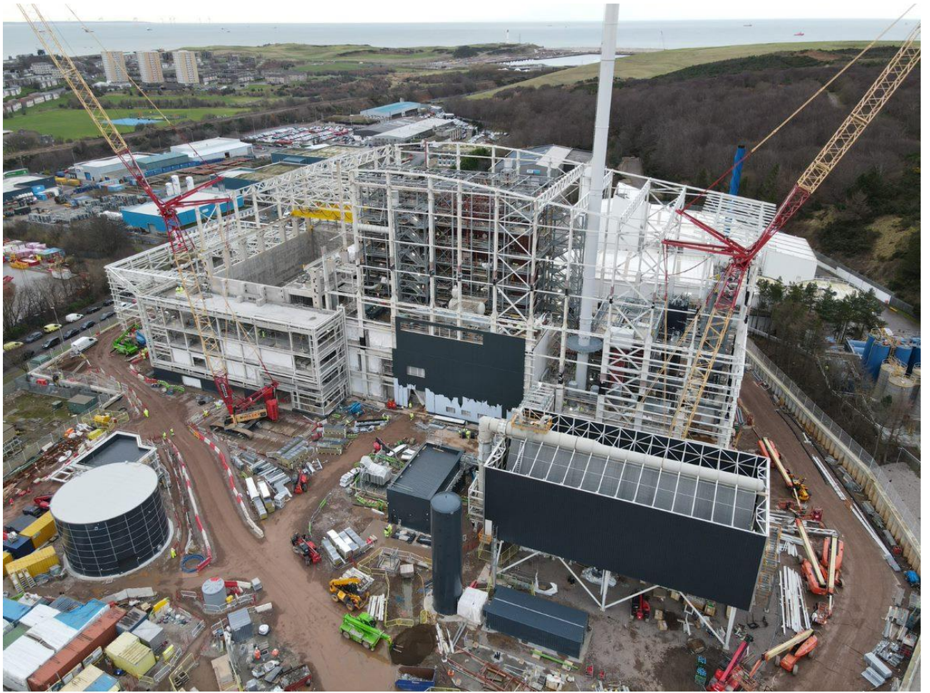
View from SW: Note Air Cooled Condenser and Fire Water Tank in Foreground
